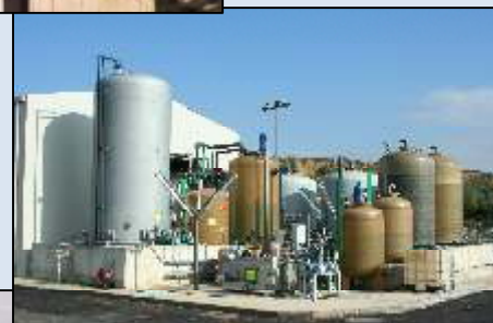
TECHNOLOGICAL SYSTEMS OF LAST GENERATION, OF DESALINATION, DRINKING WATER AND PURIFICATION
